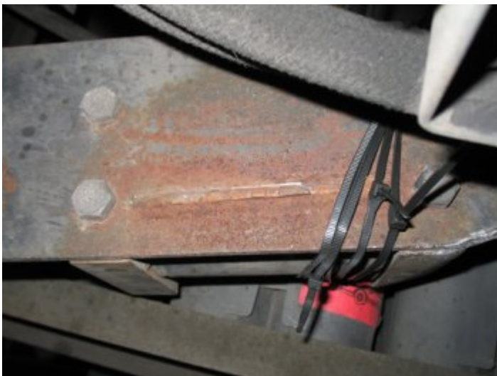
Shows where the metal fractured
