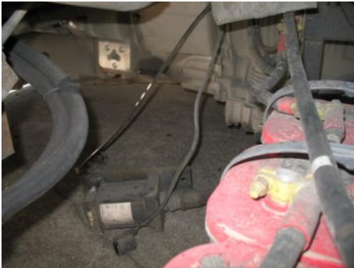
From the engine battery access door on curb side
