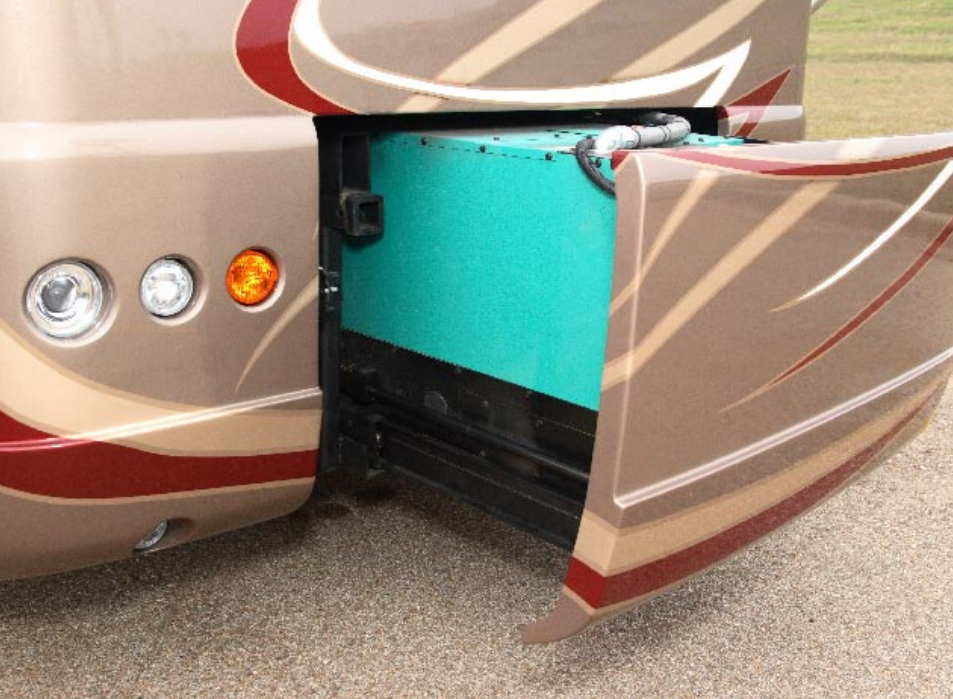
The Onan Generator is hydraulically powered for easy maintenance access.
